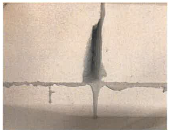
Hul i brandmur
